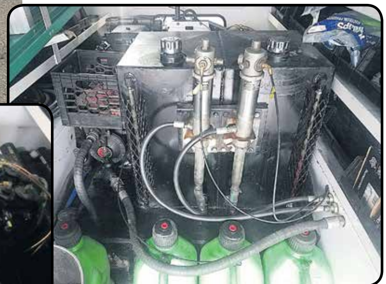
LiquidDynamics tank stores 30 gallons of antifreeze on the left side, 30 gallons of engine oil on the right side; and there's a tank across the bottom for waste motor oil.
