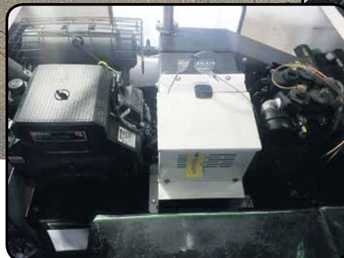
View from top of Vanair Air-N-Air shows its Kohler engine (on left), which is spaced away from the front wall to allow access to the unit's drive belts.
